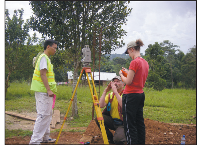
Engineering Ministries International team members (l-r) Jonathon Lee (Electrical Engineer), Patrick Cochrane (Surveyor), and Sarah Primmer (Student Intern/ Civil Engineer) survey the site of a future seniors centre in Mukono, Uganda. — photo courtesy eMi
